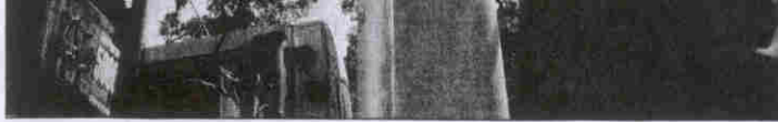
Dave McCarthy, senior radio-frequency engineer for 20/20 Communications assembles the electronic equipment for a wireless access point to be mounted on top of the Manchester tower tower Monday. The access point will be used to test signal strength in the Manchester area and is part of the Wireless Washtenaw program intended to allow wireless Internet access throughout Washtenaw County.
