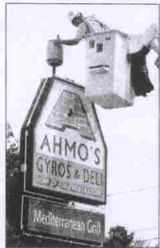
Alan Warren, the Ann Arbor News David McCarthy, radio-frequency engineer for 20/20 Communications, works on tuning the RF output signal at the wireless access point on the sign outside of Ahmo's Gyros & Deli on Huron Street in Ann Arbor.
